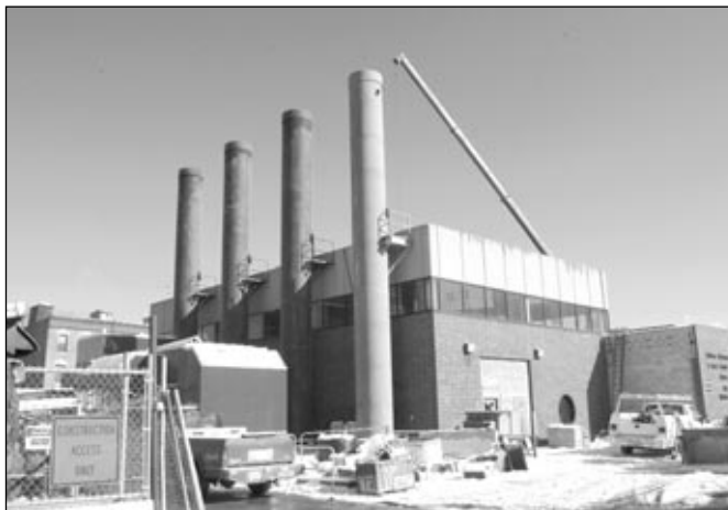
A new stack for the BWSC pump station (far right) was put into position in September 2004.
