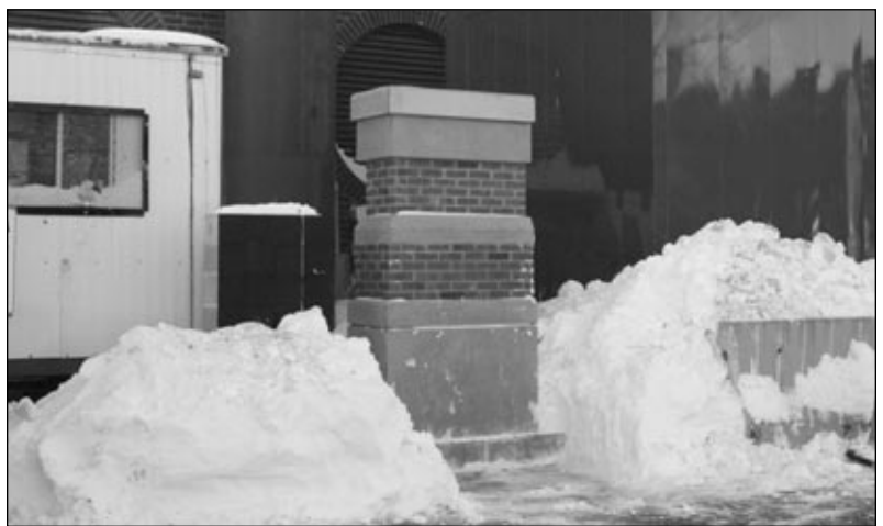
The photo above shows a mockup of the wall materials that masons will place on the exterior of the new building.
