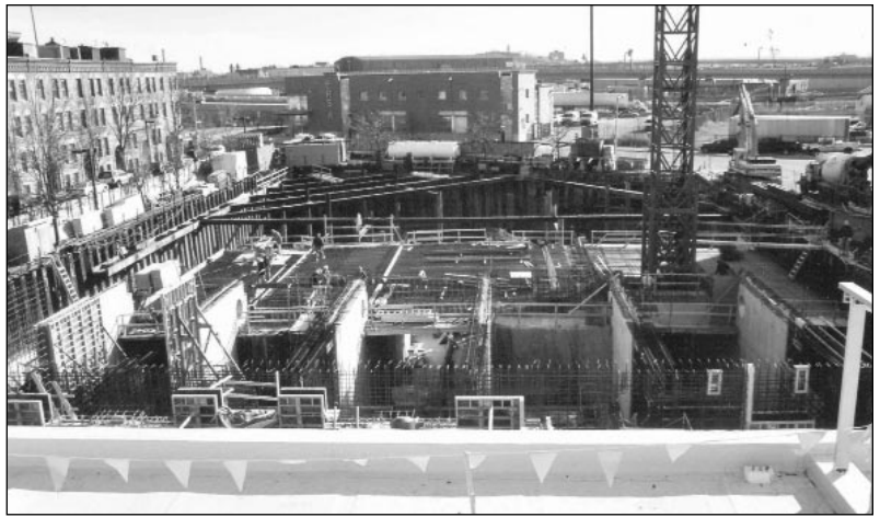
Looking east, this view of the basin construction shows interior concrete divider walls and temporary earth support framing.
