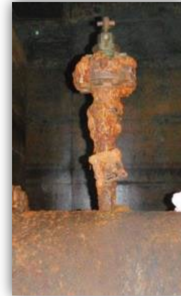
Air valve at Shaft 9A
