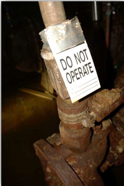
Shaft 8 PRV Chamber
