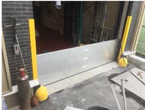
Figure 4 - Headworks Flood Barrier
