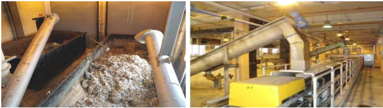
Figure 1: Grit Trailer (left) and Grit Conveyors (right) at Deer Island Wastewater Treatment Plant
