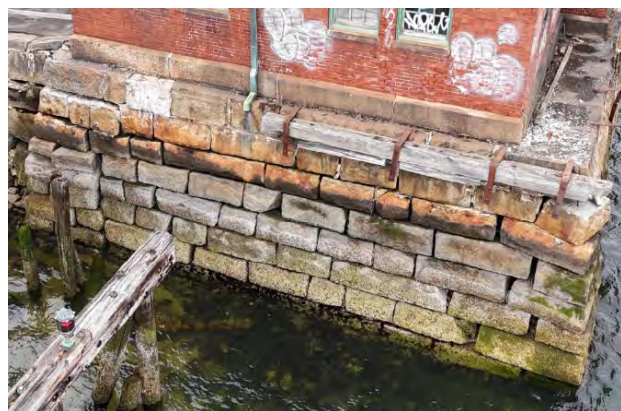
Figure 4: Deterioration at South Elevation of Seawall
