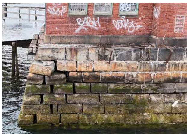
Figure 3: Localized Movement at Southeastern Corner of Seawall
