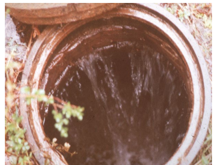
Inflow into a Sewer Manhole
