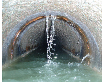
Infiltration into a Sanitary Sewer
