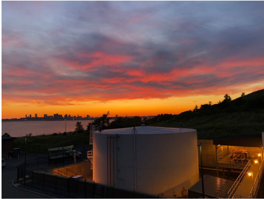
Deer Island Treatment Plant Thermal Power Plant
