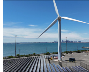
Wind turbine and solar panels at the Deer Island Wastewater Treatment Plant
