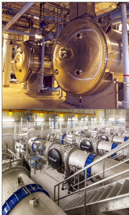
Ozone And UV Generators at the John J. Carroll Water Treatment Plant
