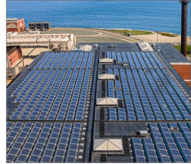
Solar panels at the Deer Island Wastewater Treatment Plant
