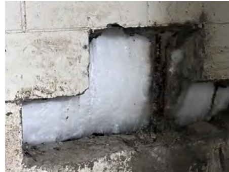
Ice Accumulation on Liquid CO 2 Piping
