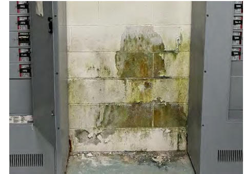
Electrical Room Damage
