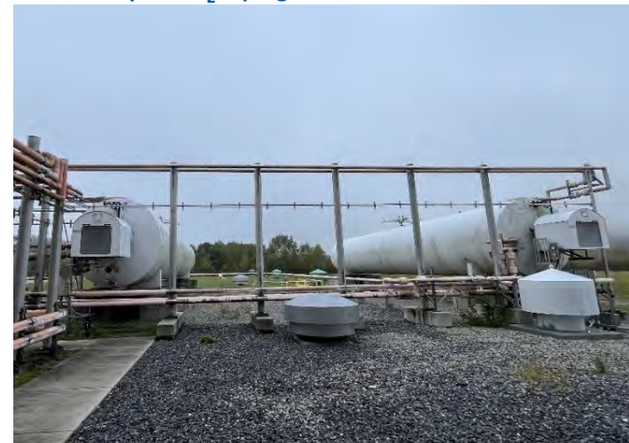
Existing CO 2 Process Piping and Storage Tanks
