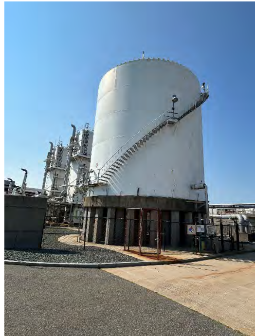
Figure 3 – LOX Storage Tank
