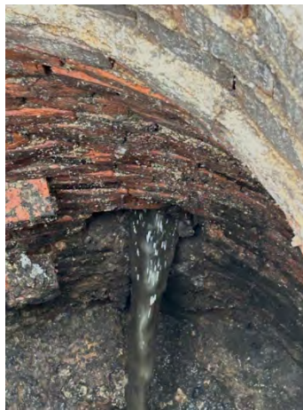
Figure 3- Garage floor drain emptying into blocked manhole
