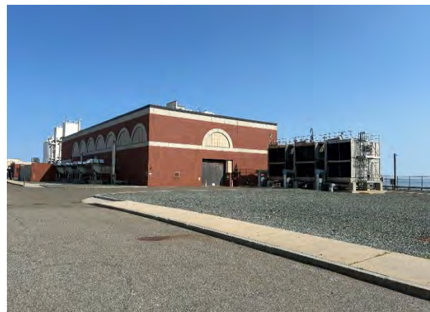
Figure 1 – Cryogenic Compressor Cooling Towers
