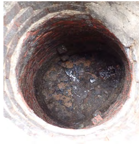
Figure 4- Closeup of blocked manhole
