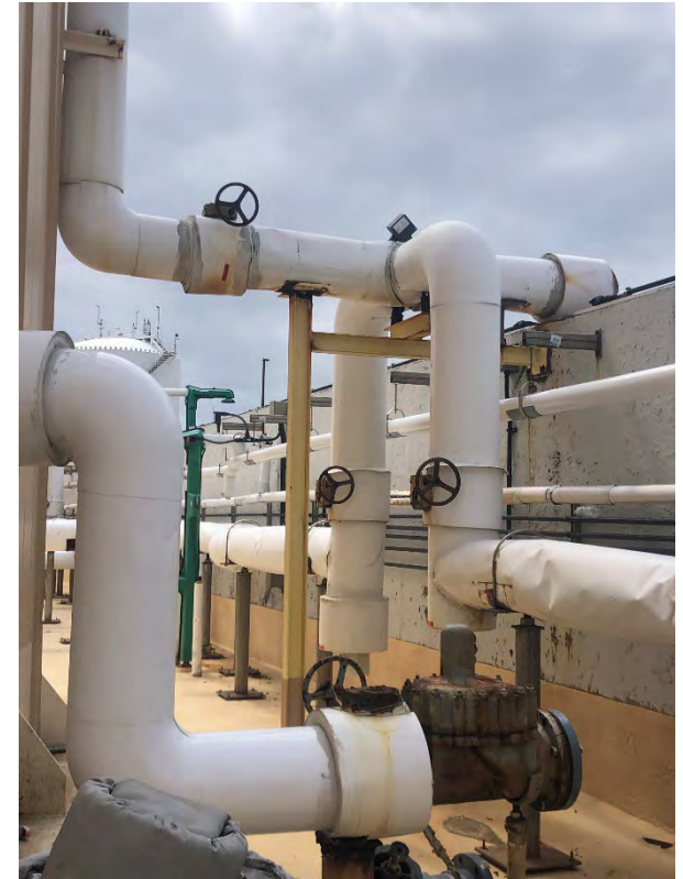
Sodium Hypochlorite Transfer and Return Lines within the Tank Containment Area
