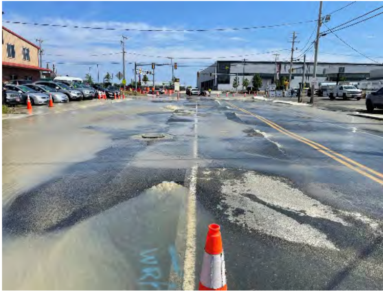
Ballard St. Road Damage
