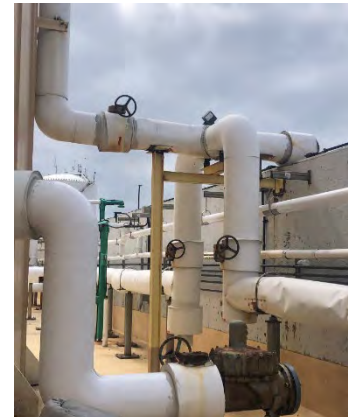
Figure 2 - Sodium Hypochlorite Transfer and Return Piping Within Tank Containment Area
