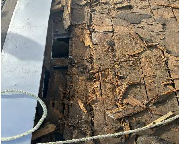
Deteriorated Wood Decking at Gillis Pump Station
