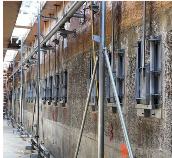
Primary Clarifier Channel Aeration System
