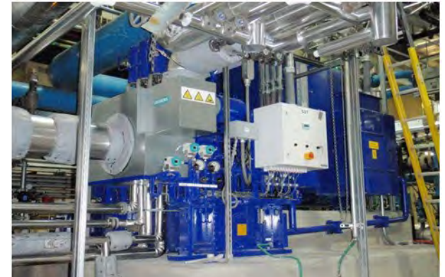
Backpressure Steam Turbine Generator
