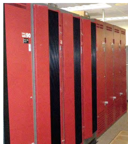
Figure 1: PICS Distributed Processing Unit Cabinets
