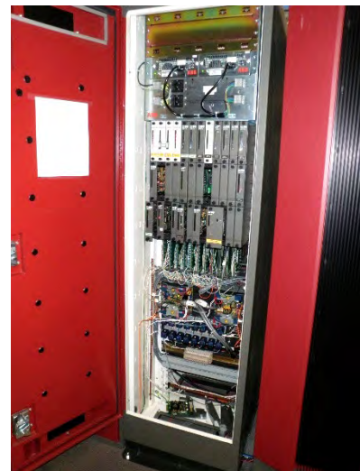
Figure 2: DPU Cabinet Showing Control Modules
