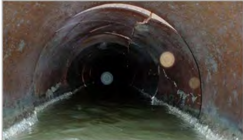
Example of Sewer Needing Rehabilitation
