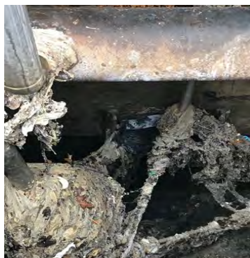
Figure 4. Rag Buildup in Process Tanks
