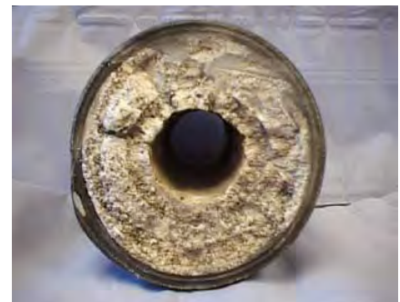
Figure 1. Struvite Blockage in Digester Overflow Piping
