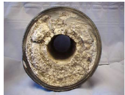
Figure 1. Struvite Blockage in Digester Overflow Piping
