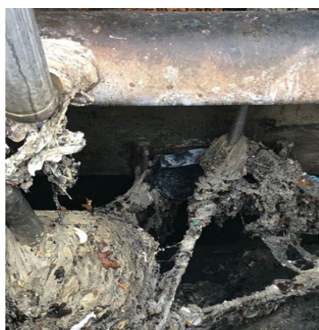
Figure 4. Rag Buildup in Process Tanks
