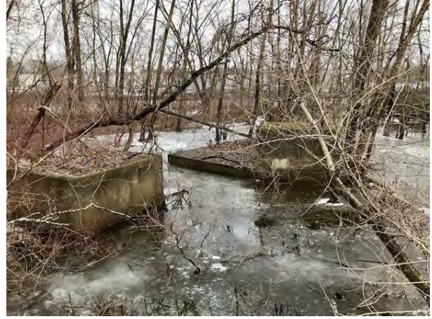
Siphon chambers subject to flooding
