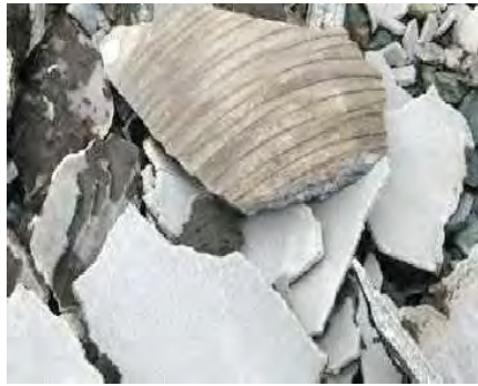
Figure 2. Struvite Buildup Removed From Pipe
