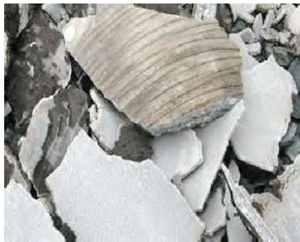
Figure 2. Struvite Buildup Removed From Pipe
