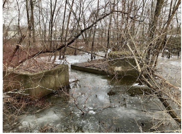
Siphon chambers subject to flooding
