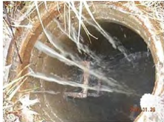
Inflow Into a Manhole During Flooding
