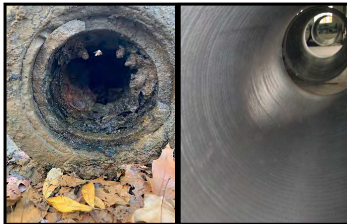
Unlined Cast Iron Main
