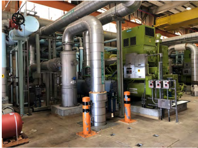
Main Air Compressor (MAC) 2A (2500 hp)
