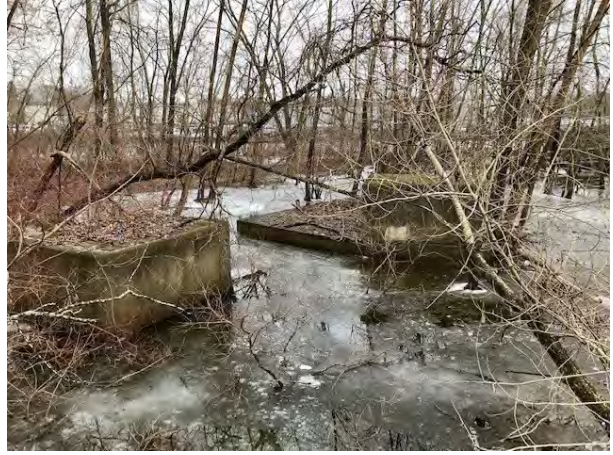
Siphon Chambers Subject to Flooding
