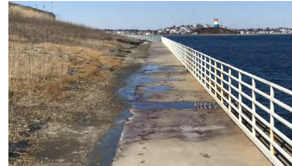
Top of wall/walkway after rain
