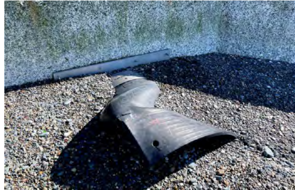
Typical duckbill valve on stormwater outfall
