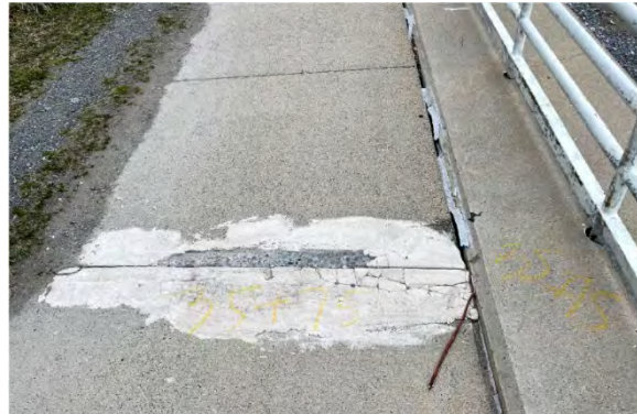
Typical spalling on public access walkway
