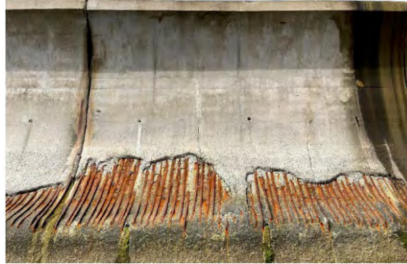
Delamination/Spalling with exposed, corroded rebar on face
