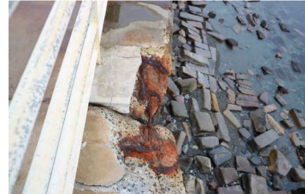
Deep spall at construction joint
