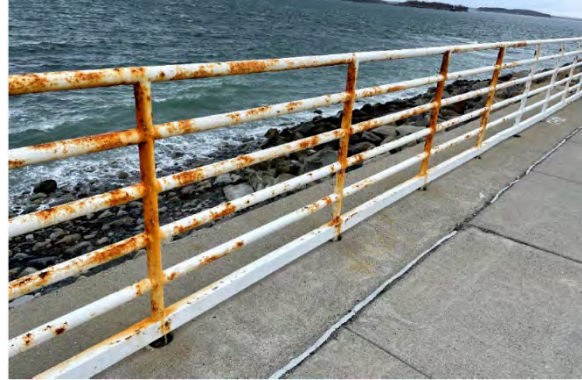
Typical corrosion to hand railing on public access
