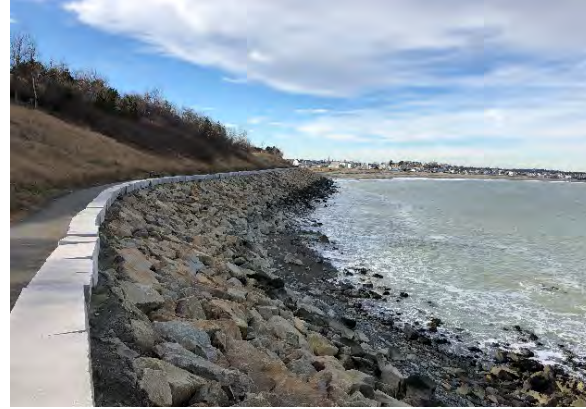
Undersized northeast revetment stone
