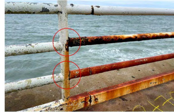
Railing separation from post
