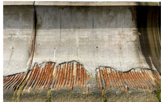
Delamination/Spalling with Exposed, Corroded Rebar on Face of Seawall
