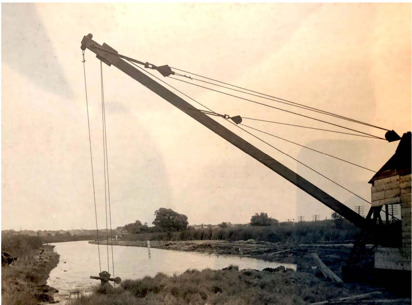
Construction of the Alewife channel with a crane dredge, circa 1909. From the Department of Conservation and Recreation, courtesy Massachusetts State Archives.
