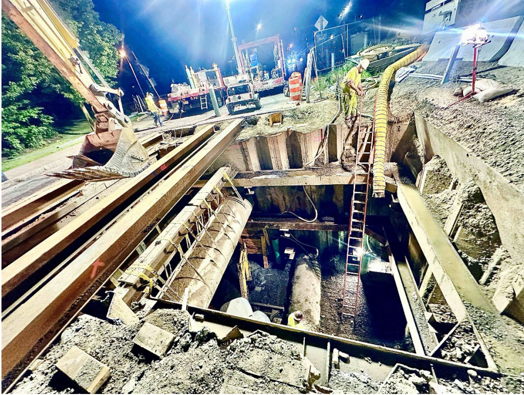
Figure B-2. Night Work Showing the Depth of the Excavation and the Construction Support Vehicles.
