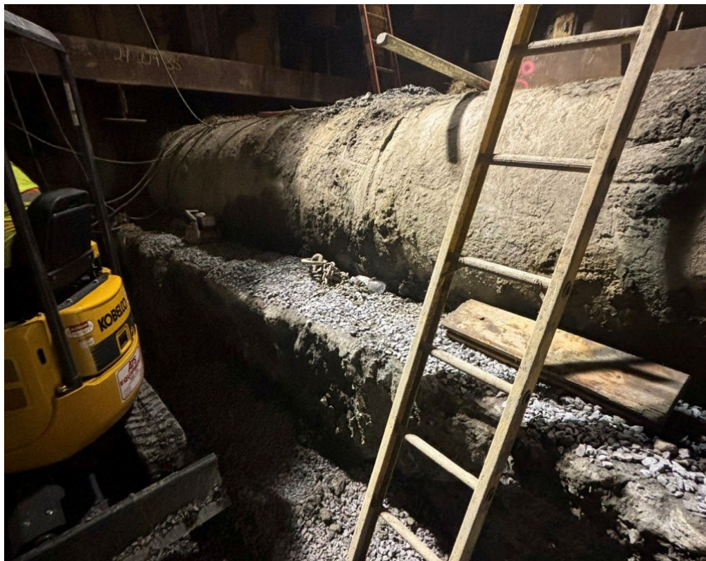
Figure B-3. Existing Slab under Section 35 to be Removed and Replaced. (Drawings for this portion of pipe were not available. Relocated pipe was shown on a hand drawn sketch.)
