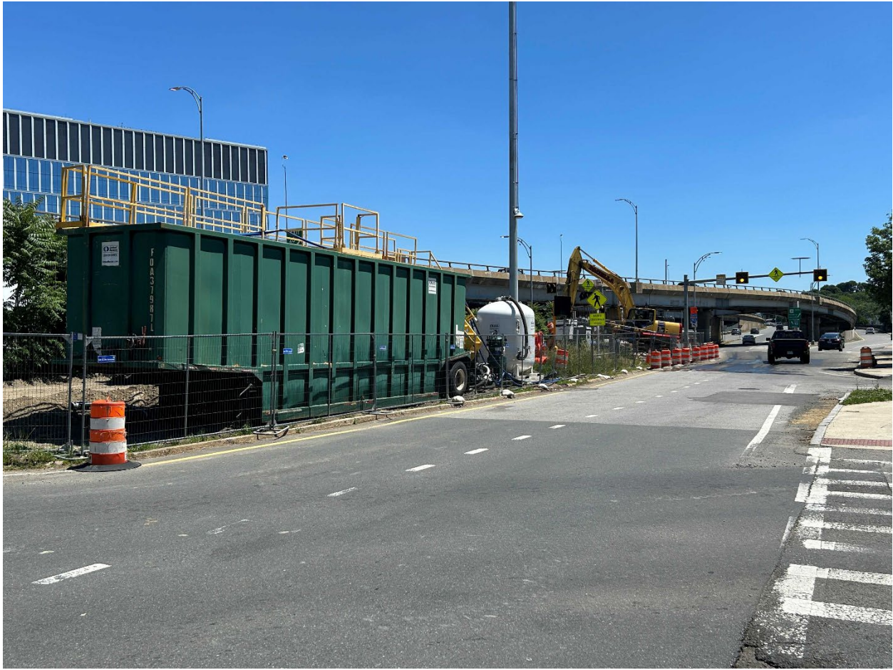
Figure B-4. Site Location Within Congested City Streets (Ramp to 93 South and Mystic Ave.)
