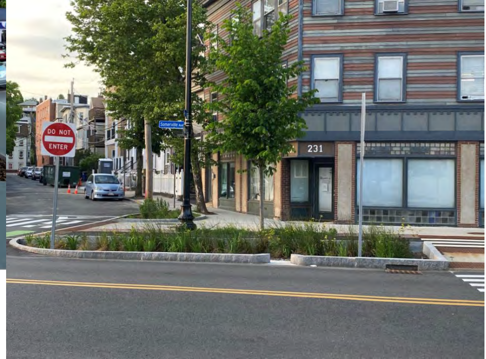
Stormwater Bump-out on Somerville Ave, Somerville (200 sf footprint, 250 cf storage)
