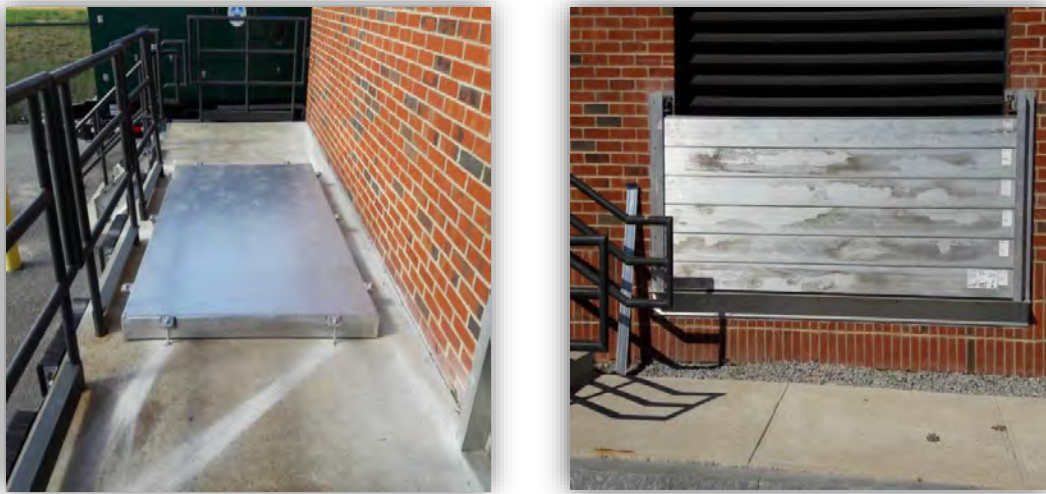
Figure 2: Braintree-Weymouth Pump Station Hatch to Screen Room (Left) and Stop Log at Entryway (Right)
