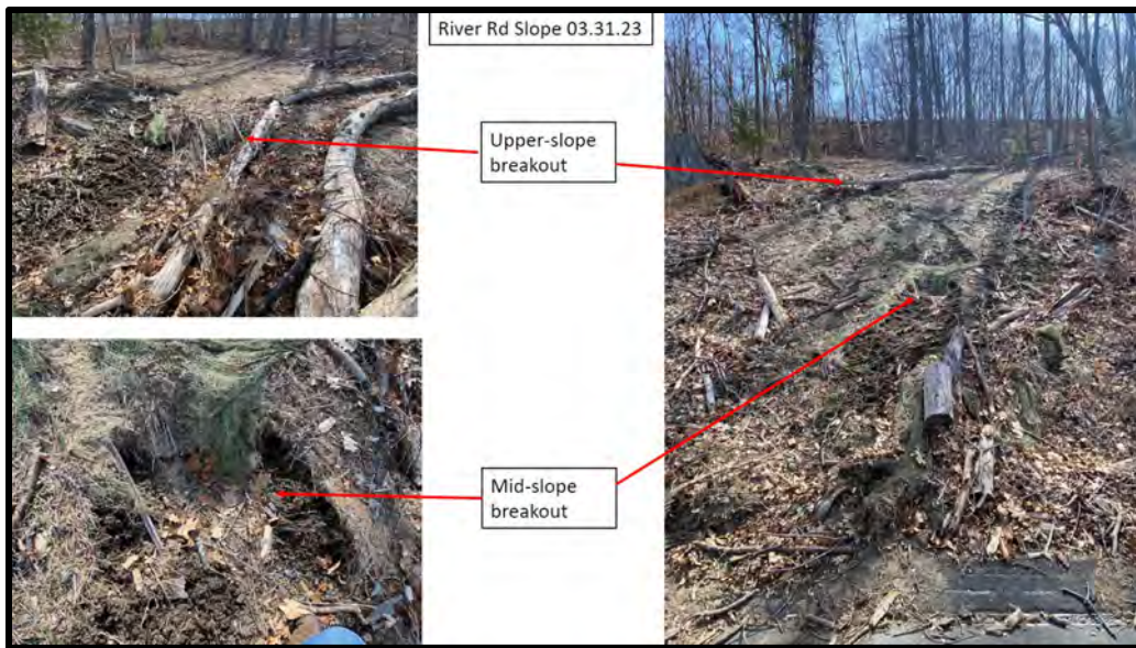
Figure 3. Groundwater breakout, Erosion and Soil Creep Upslope of River Road.
