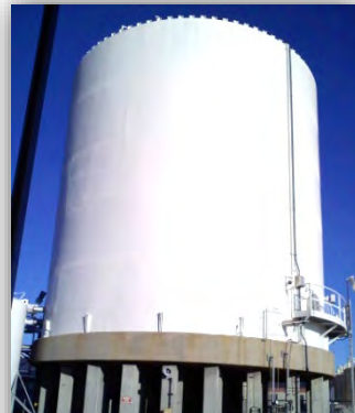
1,000 Ton Liquid Oxygen Storage
