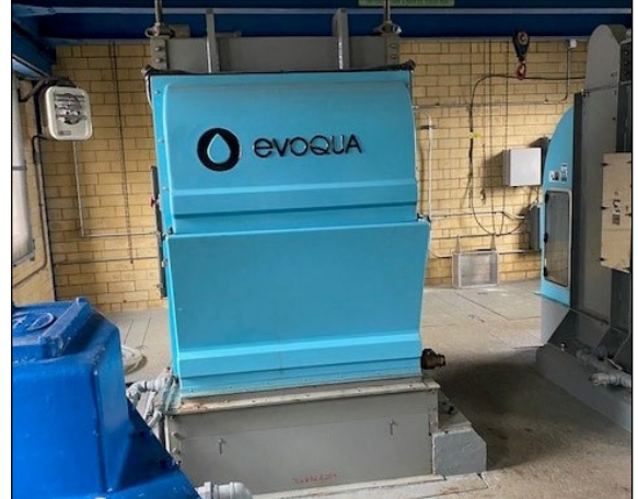
Photograph 2 – Screen washing unit inside Winsor Intake Building.
