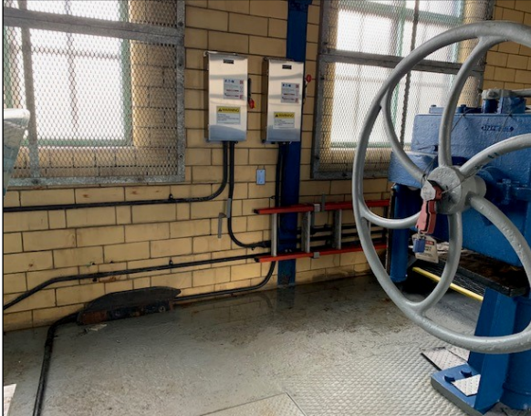
Photograph 1 – Puddled water inside north-facing wall of Winsor Intake Building.
