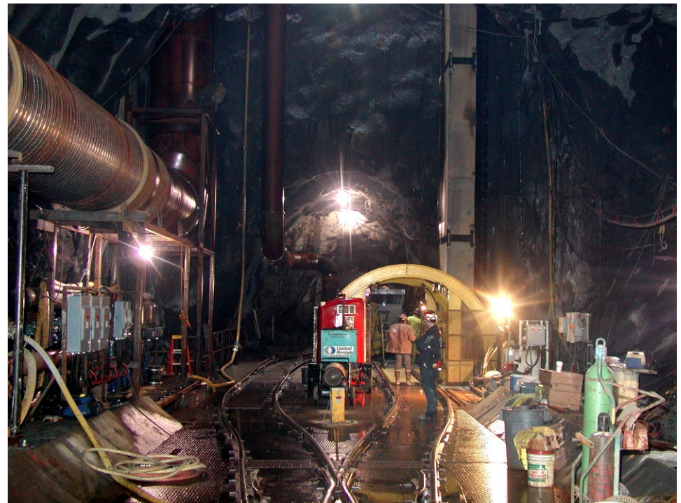
Develop base of Launching Shaft (vertical conveyor, water pumps, ventilation, TBM power)
