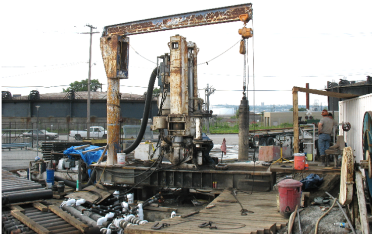
LEFT BOTTOM: Raise bore drill used to rotate and extract raise bore cutterhead to the surface (reaming the pilot hole).
