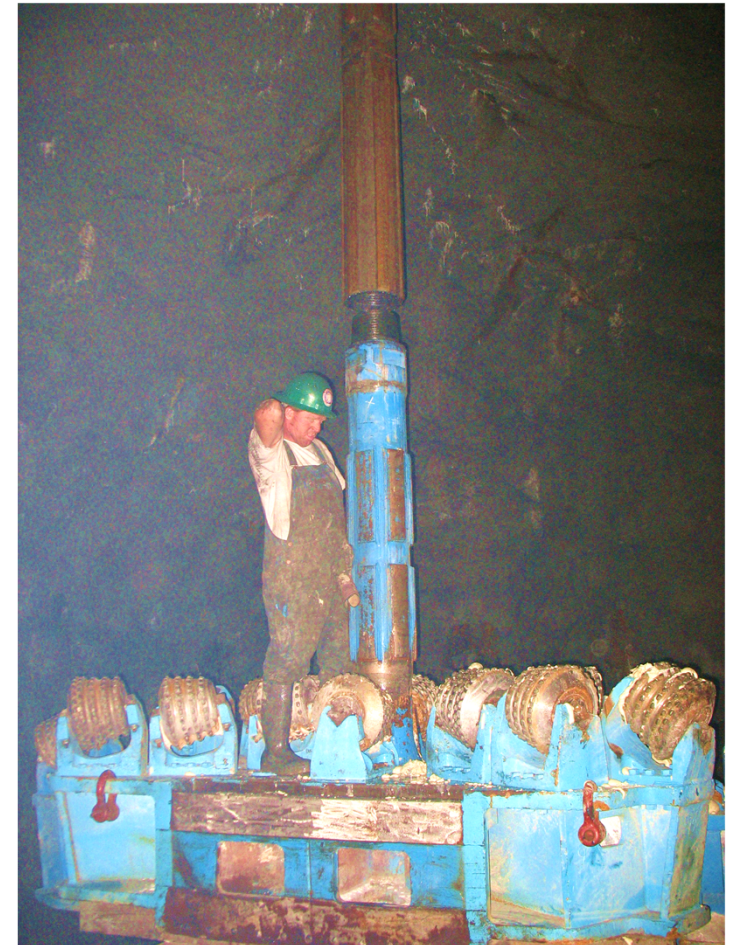
RIGHT: Worker, in tunnel, attaches raise bore cutterhead to pilot hole drill steel.
