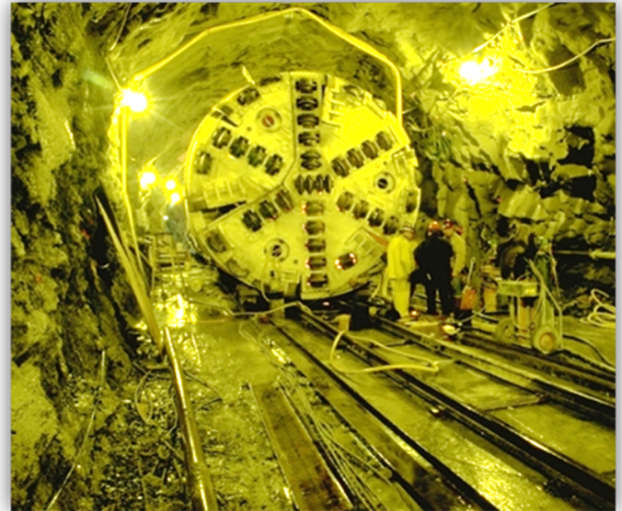
TBM Assembled on Rails moved to end of starter tunnel, and Launched
