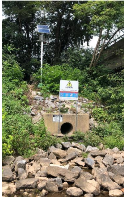
Figure 4-2. Lancaster CSO Indicator Beacon and Signage at an Outfall
