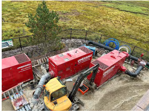
Temporary Bypass Pumping System
