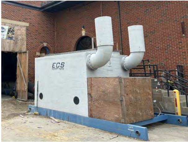
Interim Carbon Adsorber & Fan
