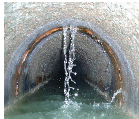
Infiltration Into a Sanitary Sewer
