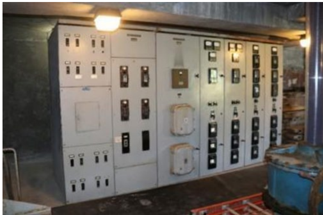
Shaft 5 - Electrical Switchgear to be replaced
