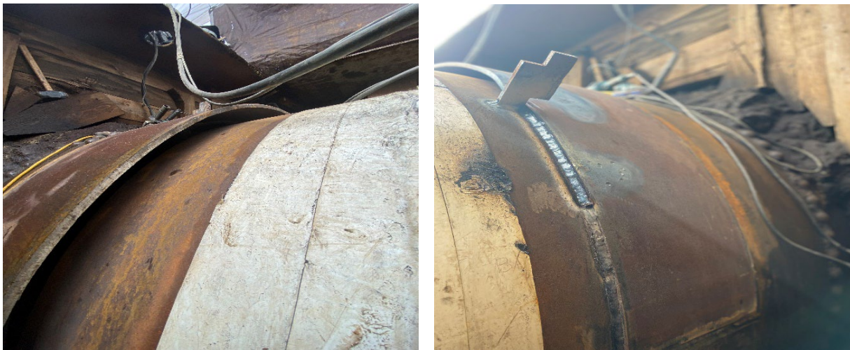
Differences in Diameter at Welding Connections
