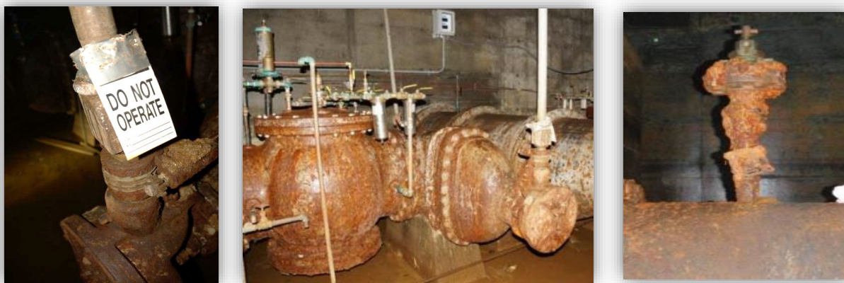
Figure 1 – Condition of Some Existing Tunnel System Valves
