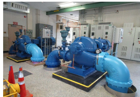
New Pumps at Commonwealth Avenue
