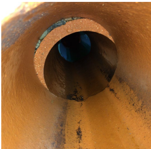
Offset Joint Detected via CCTV Inspection
