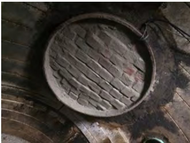
Brick and mortar bulkhead of high outlet overflow in CSO regulator CHE002-3.
