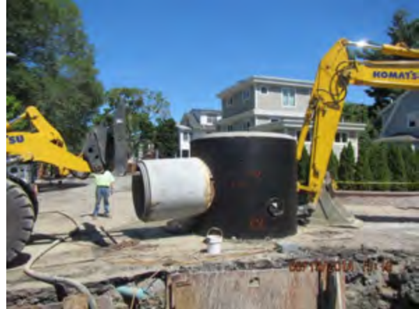
Storm Drain Manhole, Concord Avenue CAM004 Sewer Separation Contract 9
