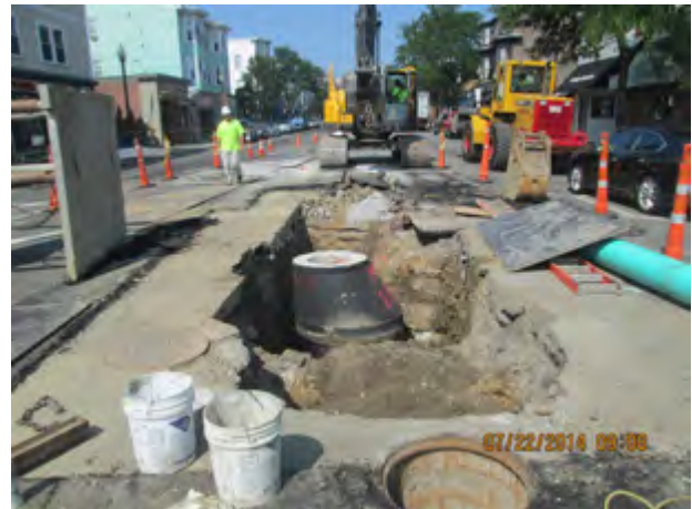
12-inch Storm Drain Installation on East Broadway Reserved Channel Sewer Separation Contract 4
