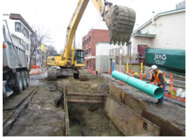
18-inch Sewer Installation on E. Third Street Reserved Channel Sewer Separation Contract 3B
