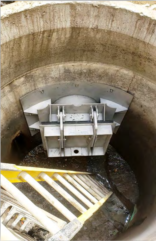
Backflow preventer installed at Waverly and Talbot Connection
