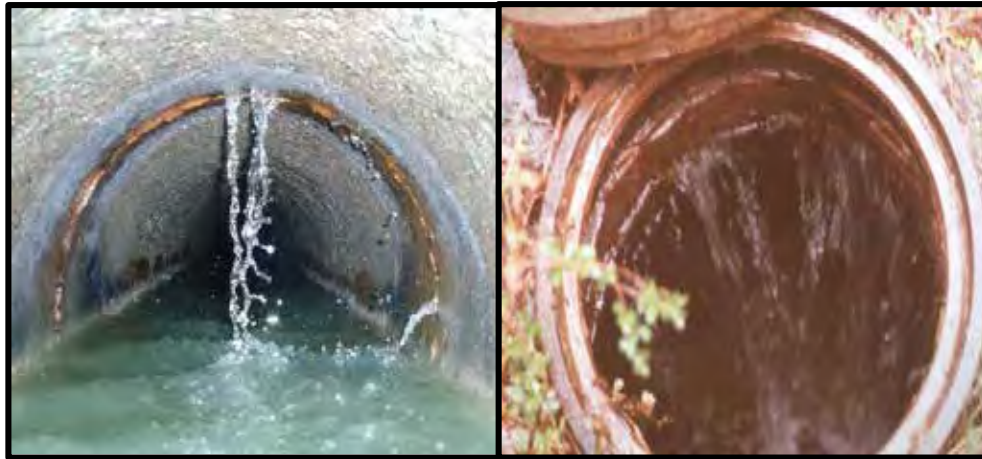
Infiltration (Groundwater via physical defects)
