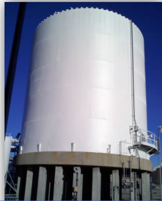
1,000 Ton Liquid Oxygen Storage
