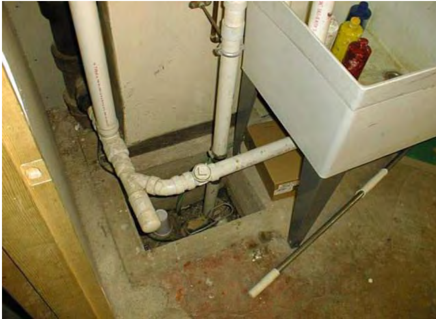
Sump Pump Direct Connection to Sewer
