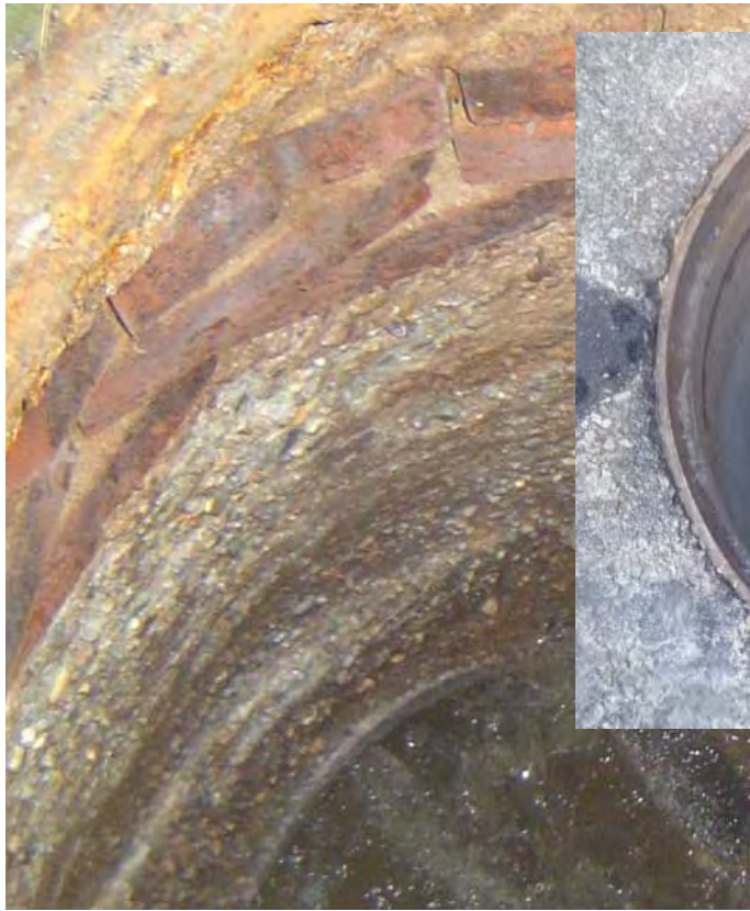
H 2 S Deterioration of Manhole
