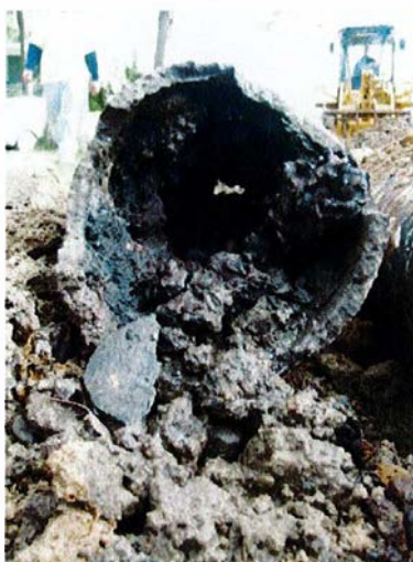
Old Unlined Cast Iron Water Main Pipe
