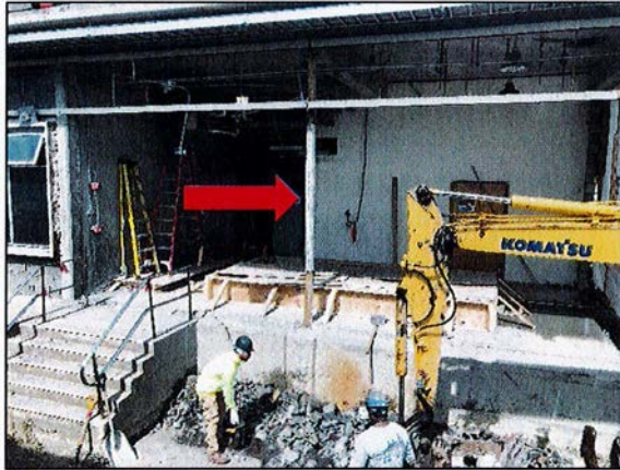
Deteriorated Column Requiring Reinforcement
