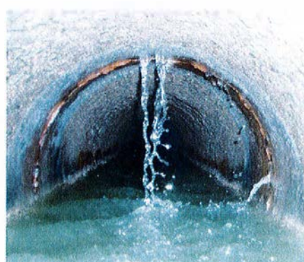
Infiltration into a Sanitary Sewer
