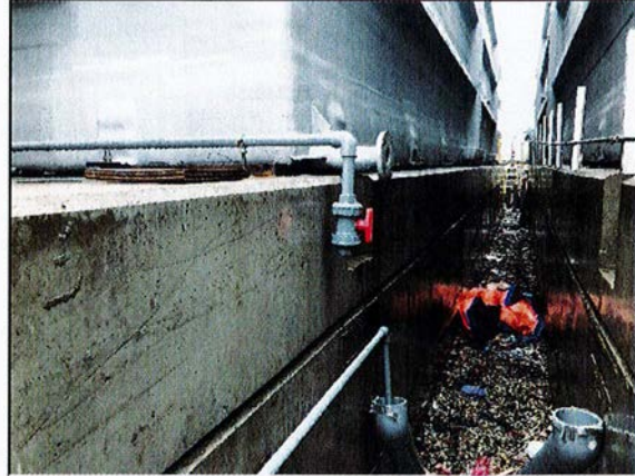
Buried Condensate Drain Lines
