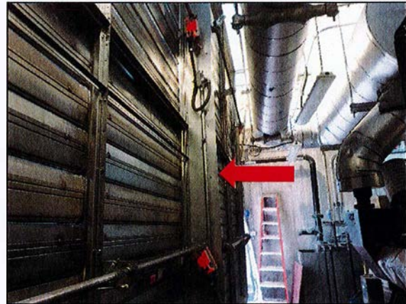
Staggered Dampers around Reinforced Column
