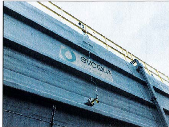
Sensing Lines for Differential Pressure Gauge
