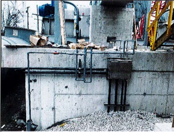
Additional Traps Assembly at Odor Control Fan
