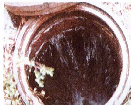
Inflow into a Manhole during Flooding
