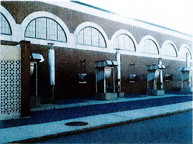
Air Compressor Building with Air Intake Ducts
