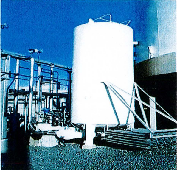
Six-Ton Liquid Oxygen (LOX) Transfer Tank
