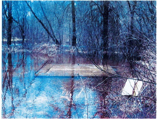
Flooded siphon chamber
