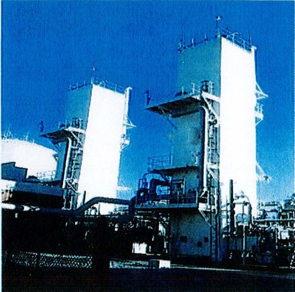
1,000-Ton LOX Storage Tank (in background) and two "Cold Boxes"
