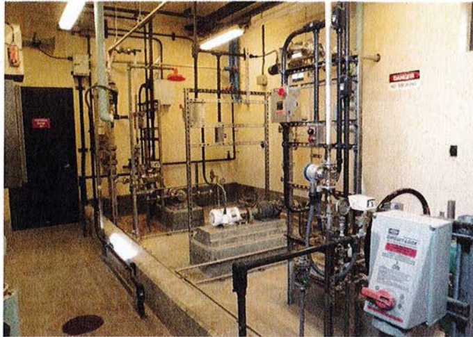
South System Hydrogen Peroxide Pump Room
