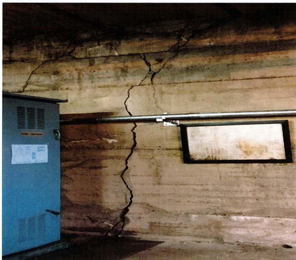
Photo 2 Bastion Wall Crack
