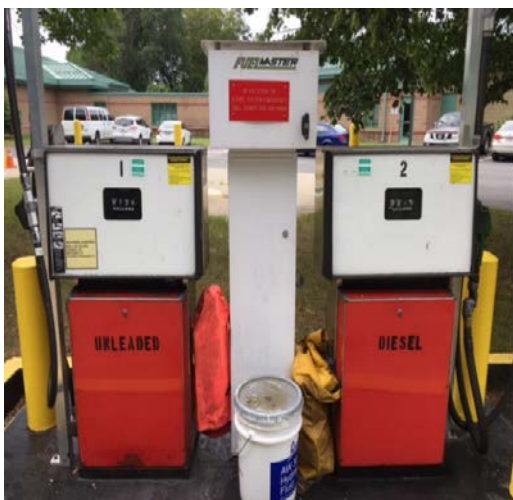
Figure 3- Southborough Fuel Pumps
