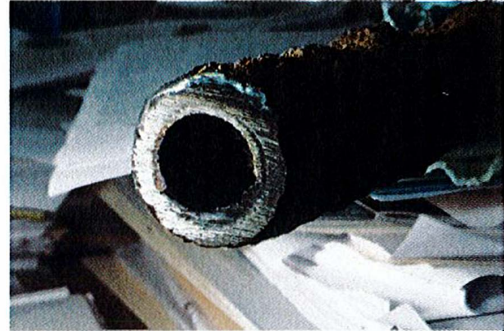
Sample photo of lead-lined steel water service line removed in Quincy
