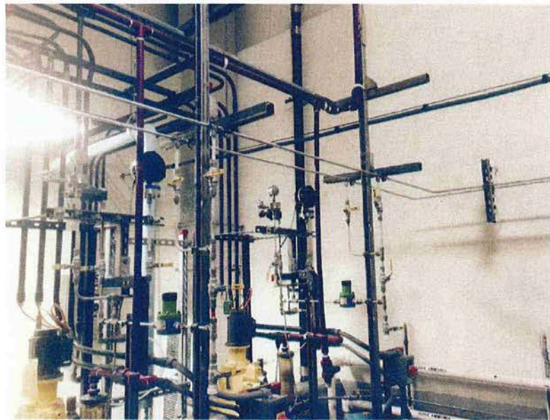
Carroll Treatment Plant ammonia system piping improvements
