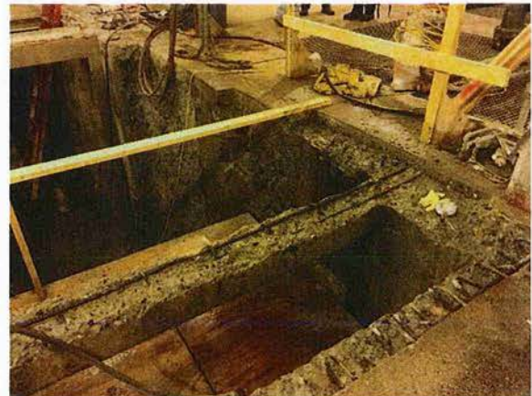
Repair of poor concrete at new catenary screen opening. Note the irregularities in the side wall surfaces
