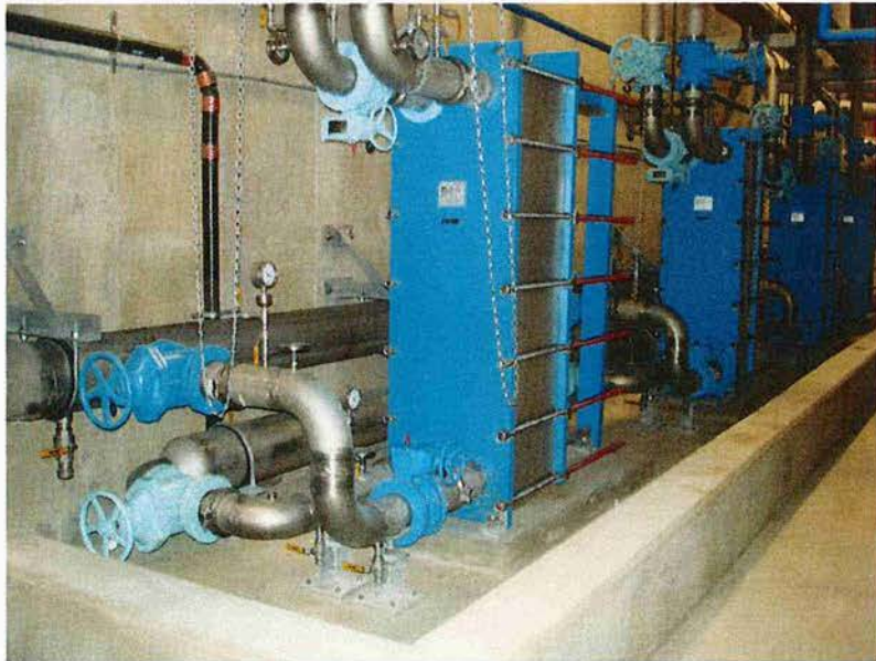
Heat exchangers for ozone generators closed-loop cooling system
