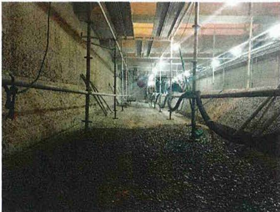
Deteriorated concrete in process channel below water line
