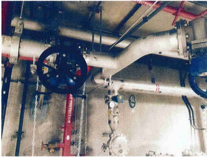
Second oxygen feed pipe to the ozone generators for redundancy
