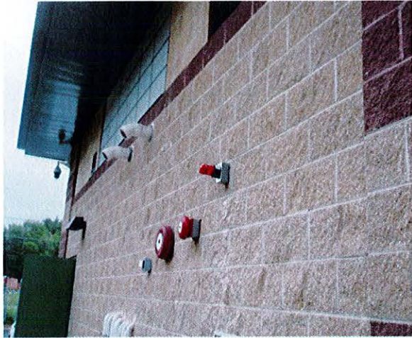
Fire Alarm Strobe on outside of the building
