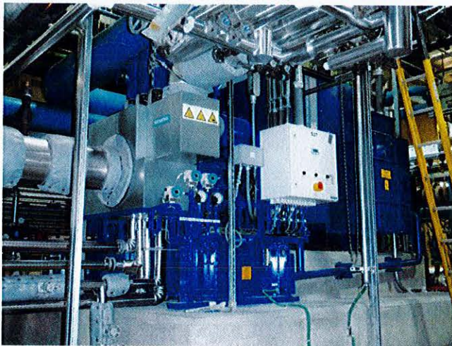
Fig. 3: 1.2 MW Back-Pressure Steam Turbine Generator
