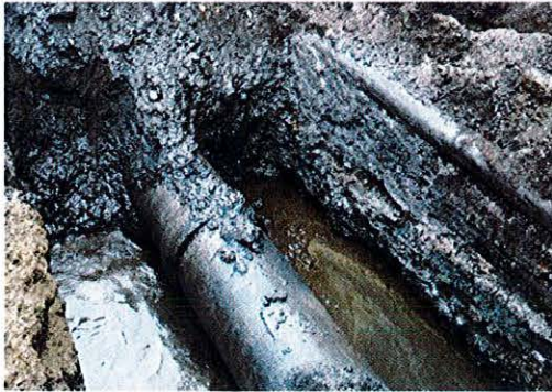
Oil in Test Pit for Storm Drain
