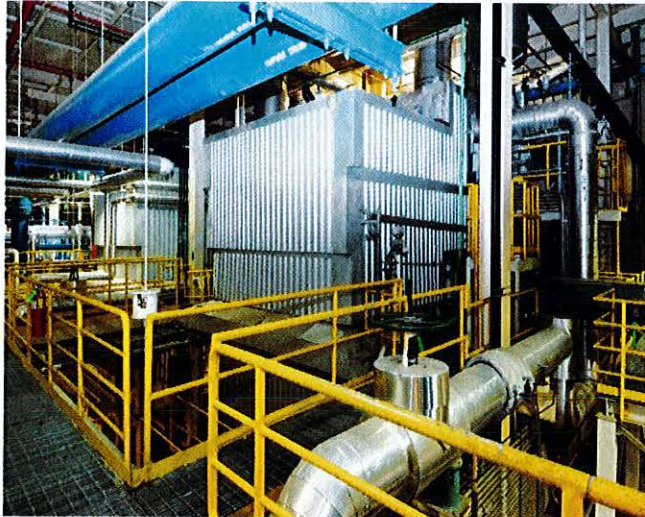
Fig. 1: Two High-Pressure Steam Boilers
