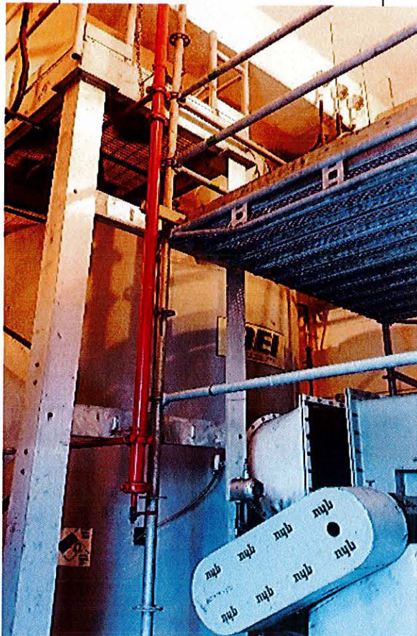
Figure 2 – Manual Screens in lower Influent Room
