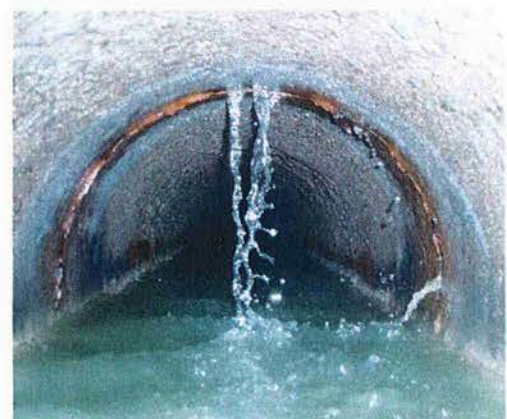
Infiltration in a Sanitary Sewer
