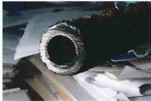
Lead-lined service line, similar to lines Quincy found during their project
