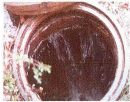
Inflow into a Manhole
