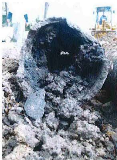
Old Unlined Cast Iron Water Main Pipe
