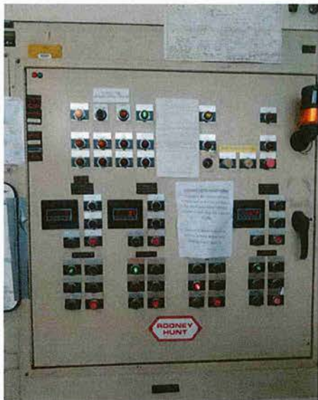
Sluice gate control panel – front
