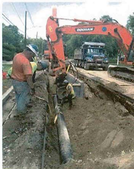
Summer Ave., Reading – Installing 36-inch MWRA water main and 12-inch Town of Reading water line
