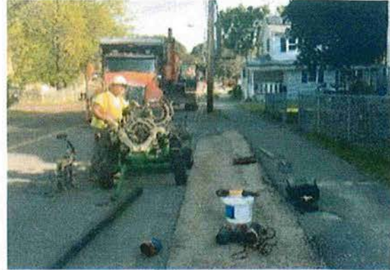
Oak Street, Stoneham – Fusing temporary water bypass piping for homeowners while main water supply is out during 48-inch installation
