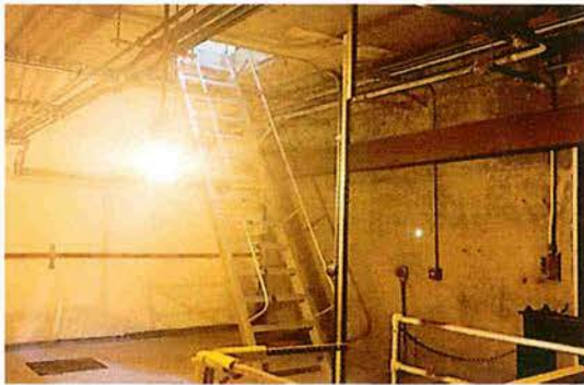
The existing opening must be enlarged for the new stairwell. Structural additions are required to support the roof
