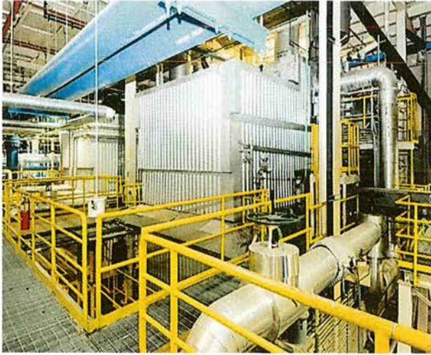
Two High-Pressure Steam Boilers
