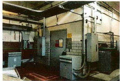
Electrical gear that is in conflict with the new switchgear room
