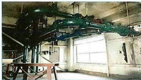
Grit & Screenings piping in new third floor mechanical room
