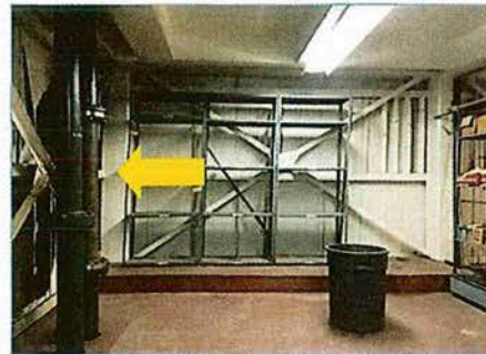
Grit & Screenings piping in new second floor electric room
