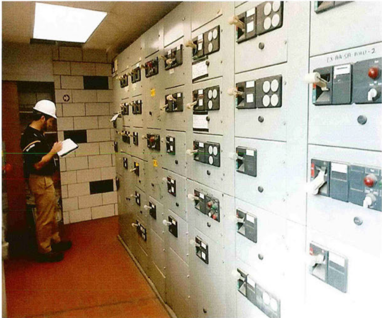
Figure 2-NMPS Motor Control Center
