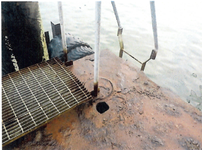
View of a small hole on floating dock no. 1 prior repair during summer of 2015.
