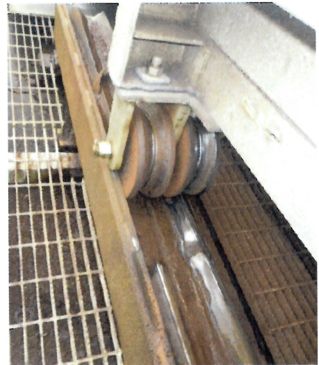
View of a damaged track for the gangway on floating dock no. 1.
