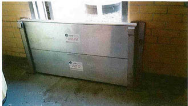
Figure 3: Stoplogs At The Alewife Pump Station
