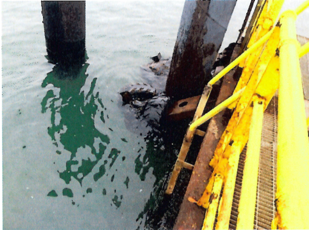
View of the damaged collar on floating dock no. 2
