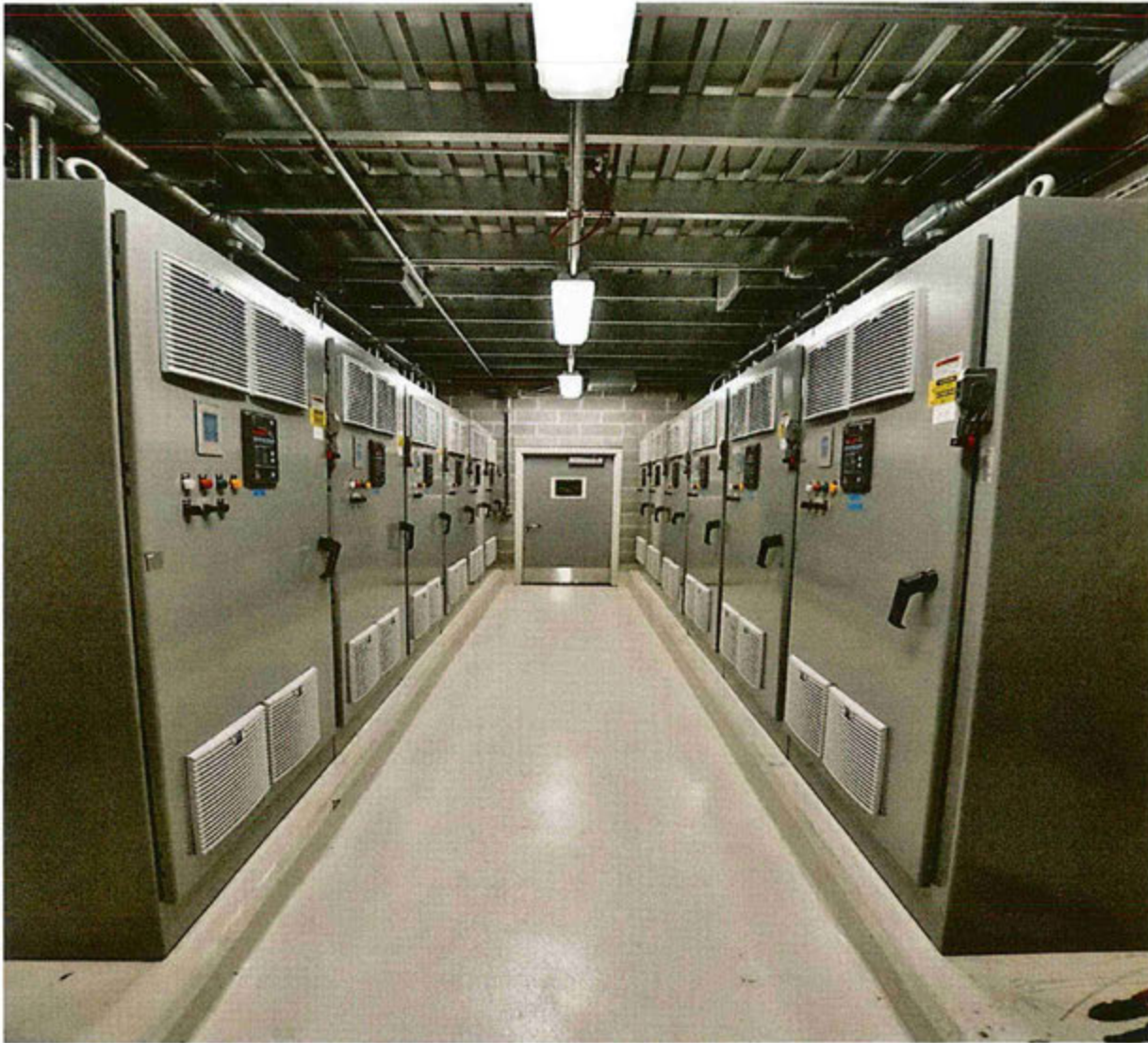
Deer Island Wastewater Treatment Plant New Reactor VFD Room
