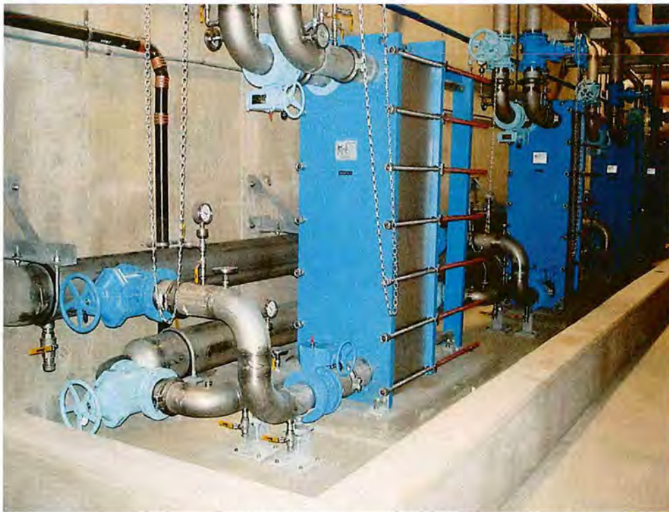
Heat exchangers for ozone generators closed-loop cooling system
