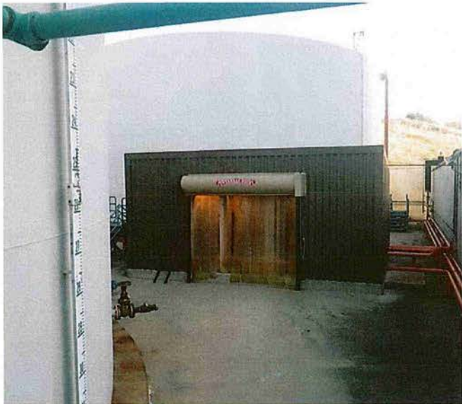
Fuel Oil Skid Enclosure
