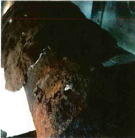
Exterior rust and corrosion of the Pipe under the bridge, 2015
